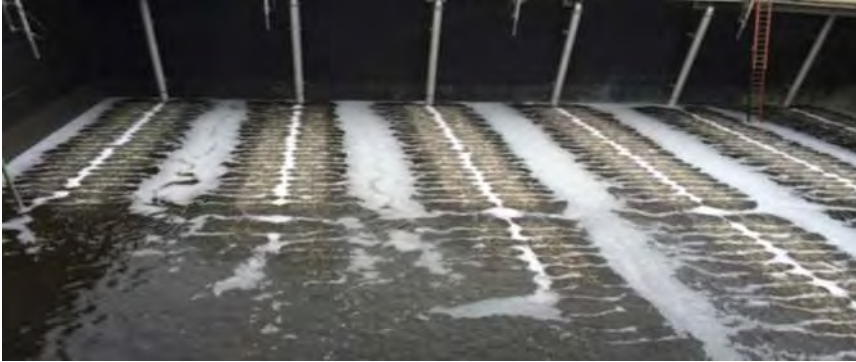
Improper Leveling of Aeration Grids in Aeration Basin
