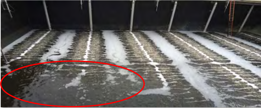
Improper Leveling of Aeration Grids in Aeration Basin
